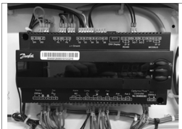
Picture 4 : Normal wiring
